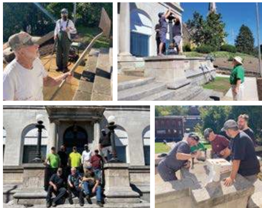
Members of the Cumberland Scottish Rite, Blue Lodges, and other organizations that call the Cumberland Masonic Temple home have been busily making improvements, small and large, to the Temple. Volunteers are pictured here working on landscape improvements and making necessary repairs to century old lighting fixtures at the Temple.
